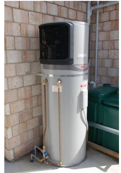
Heat pump hot water system
