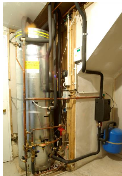
In both these cylinders you can see that the pipes moving hot water are lagged to prevent heat loss.
