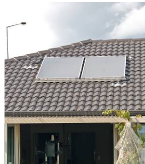
The Waitakere NOW Home panels were only installed at 20° in line with the roof. It should have sat at 37°
